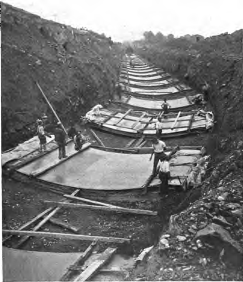
PLATE 129.—Contract 15. Laying Alternate Blocks of Invert for Cut-and-cover Aqueduct. Concrete mixed at stationary plant, hauled on cars and placed by locomotive cranes. Blaw steel profiles used, surface rolled with steel shafting. On this contract excavation and invert were kept far in advance of arch.
